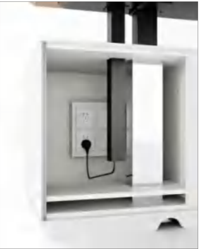
插座取电特写 Close-up of power taking from socket
